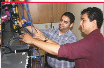
900 Building CISCO Computer Lab
