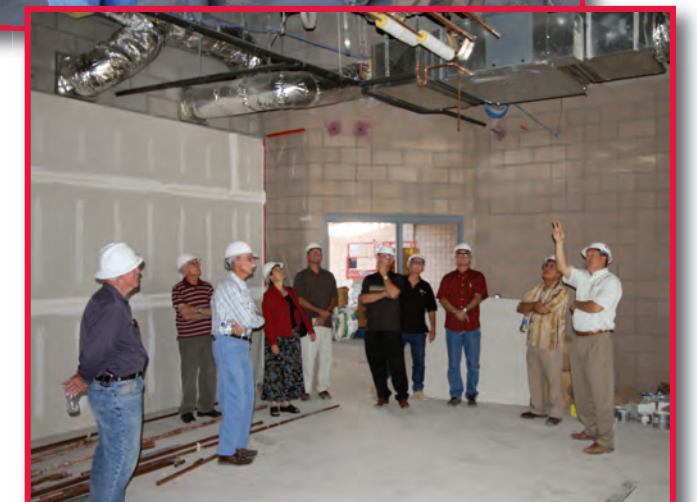
Jimmy Sanders of Sanders, Inc. conducting a tour of new science building with Oversight Committee members.
